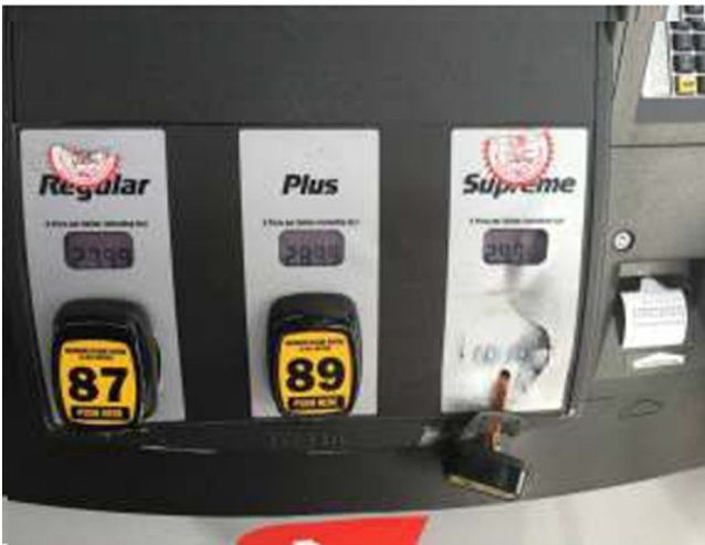
Figure 1 - This $578.00 repair was turned in as a $24,568.00 total loss replacement.
