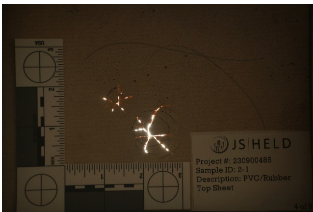
Figure 6 - Light passing thorough fully developed fractures in membrane roofing, observed with use of high intensity backlighting, and registered by long-exposure photography.
